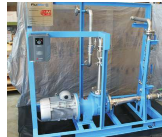
Bekaert China application for waste water transferring
